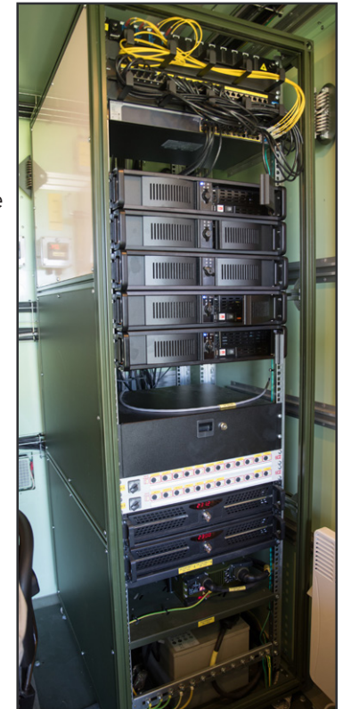
MGCS server rack
